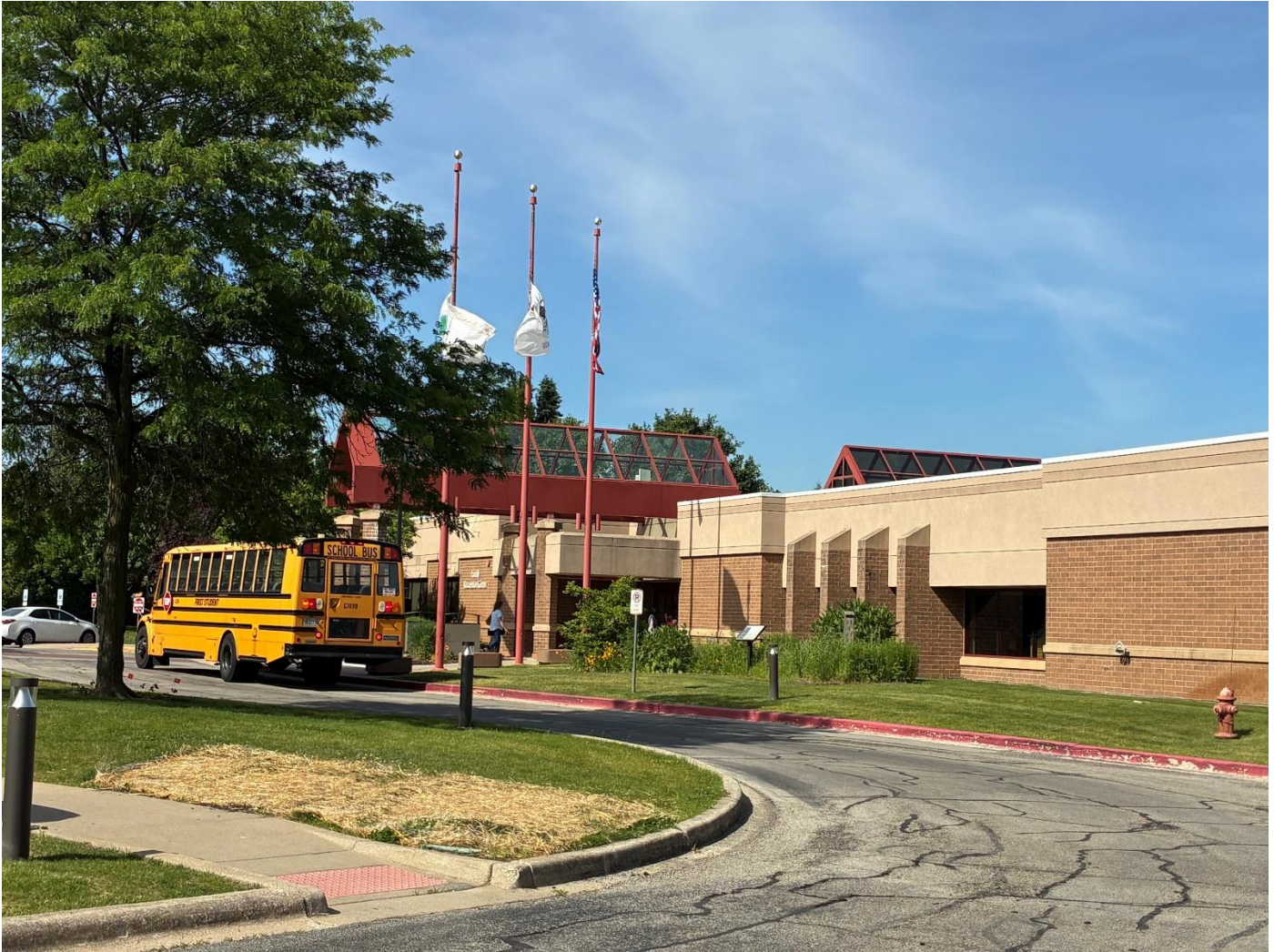
EIFS painting/repairs, awing (both sides), skylight, three flag poles, window trim.
