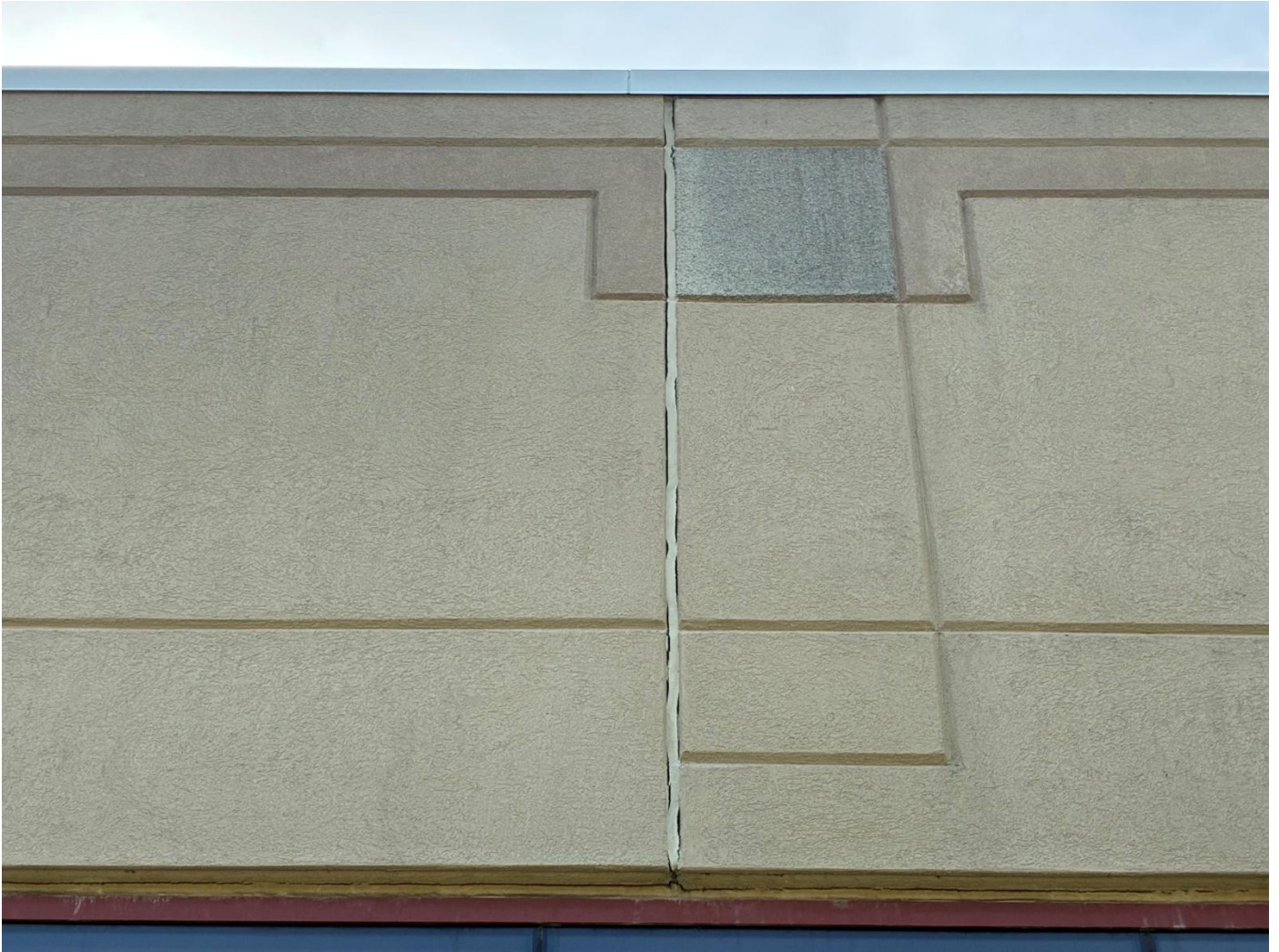
Reference photo for failed caulk joint.
