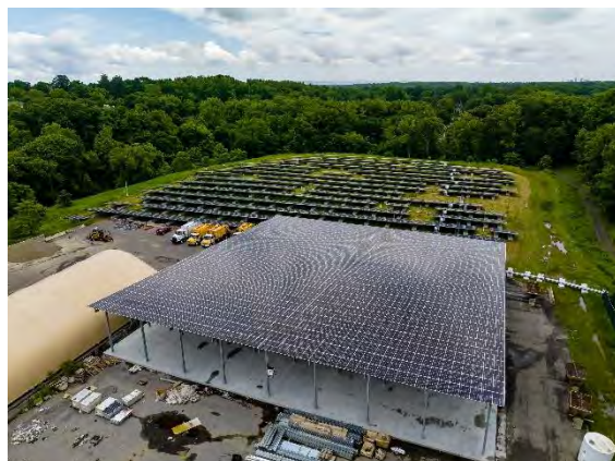
Figure 8. Gedney Way Recycling Facility floating foundation solar canopy on a landfill
