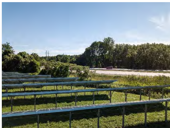
Figure 10. 4.6 MW ground mount solar project in Niskayuna, NY
