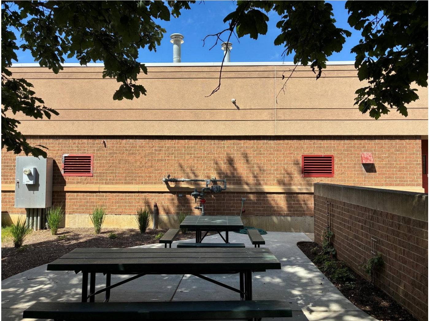
EIFS painting/ repair and three vents.
