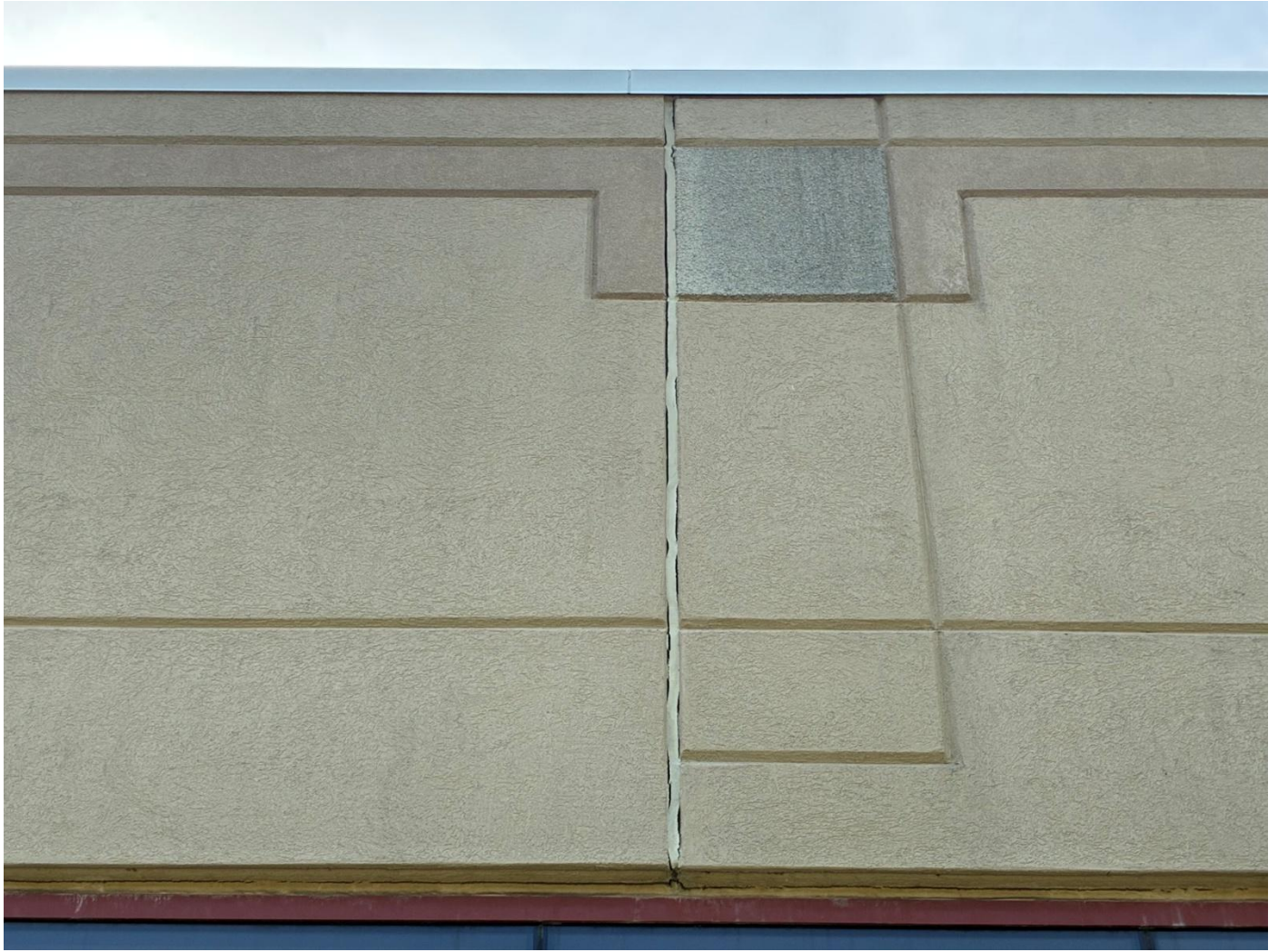
Reference photo for failed caulk joint.
