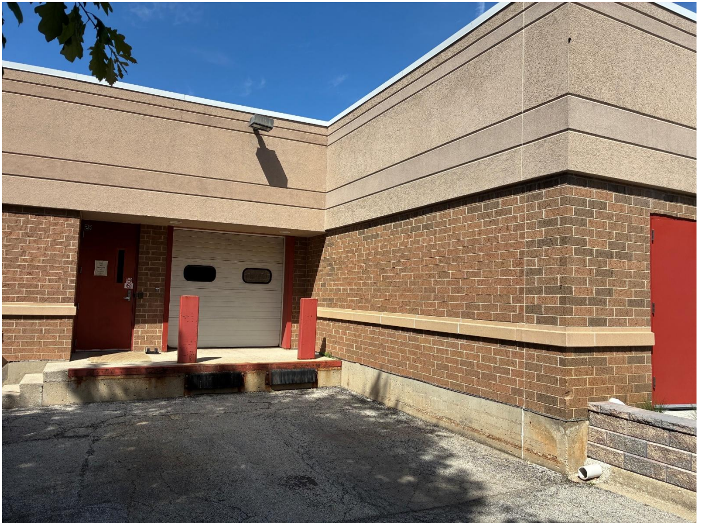
EIFS painting/ repair, door (#2B), garage door trim, two bollards, and truck stop.
