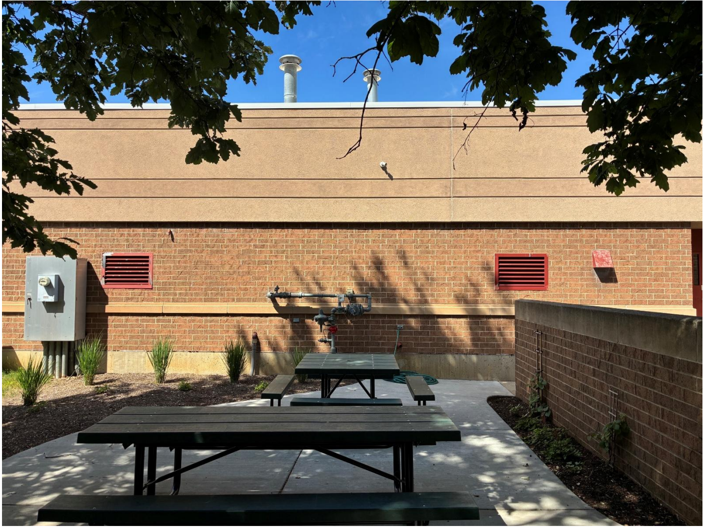
EIFS painting/ repair and three vents.
